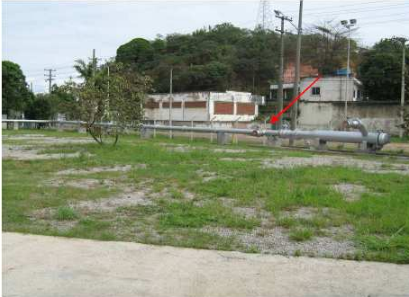
Photo A – 14” Loop red arrow indicating location of the Magnetic Filter
