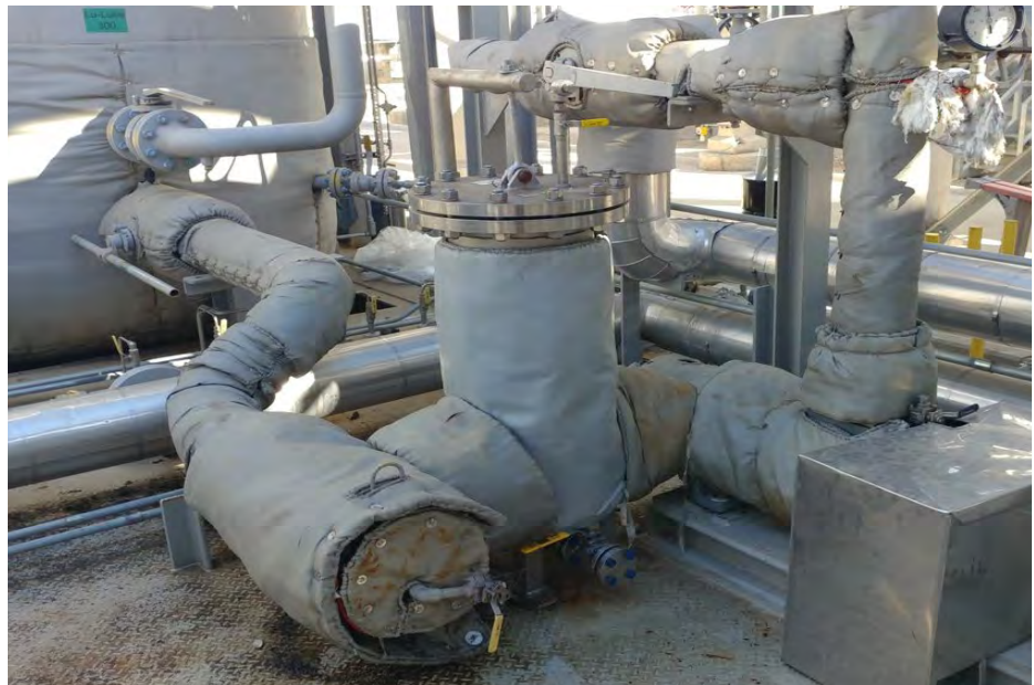
Compressor lube oil system with magnetic filtration installed.
