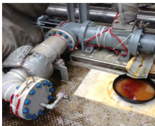
Compressor lube oil system before magnetic filtration.
