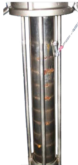
CONTAMINATION CAPTURED BY THE MAGNETIC FILTER ELEMENT
