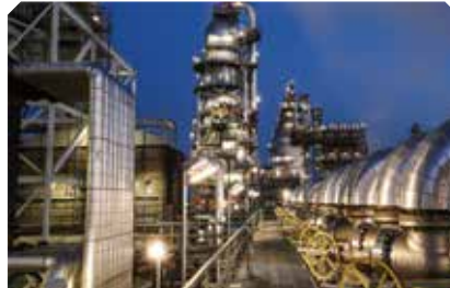
OIL & GAS PLANT
